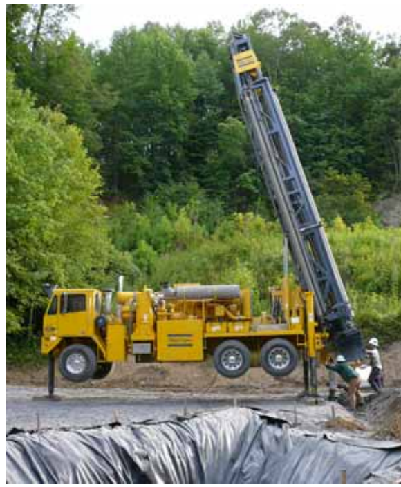
Drilling Monitor Well (BD-114M2) at the Central Appalachian Coal Seam Project site in Russell County, Virginia.
